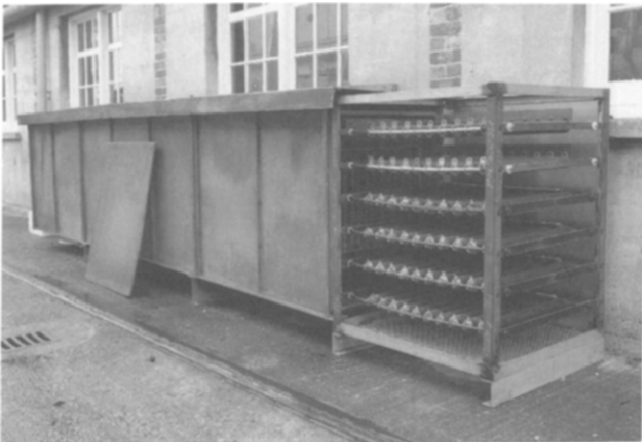
Fig. 4. Photograph showing the partially uncovered high-power resistor load bank; the load bank comprises 255 0.4 \Omega resistors.
